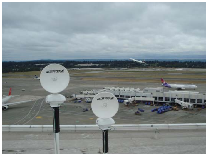
Accipiter ® radars at Seattle-Tacoma International Airport
