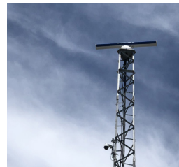
Accipiter® NM1-8A Radar Surveillance and Camera System, located at Port Dalhousie, Ontario, Canada
