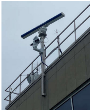
Relocation of Radar from the Roof top to Wall Mount with Addition of Axis Q8742-LE Bi-spectral Camera
