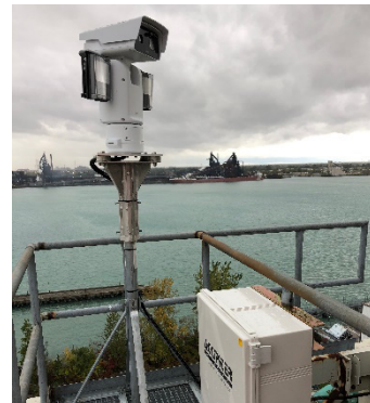
Axis Q8741-LE Bi-spectral PTZ Camera Installation at Brighton Beach Power Generating Station
