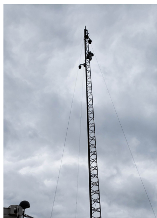
Axis Q8741-LE Bi-spectral PTZ Camera Installation at Lafarge Holcim Dock
